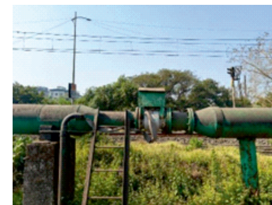
Fig: Incoming water meter photograph
